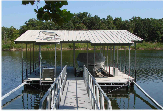
Solar panel mounted on single-slip dock in the Ozarks
